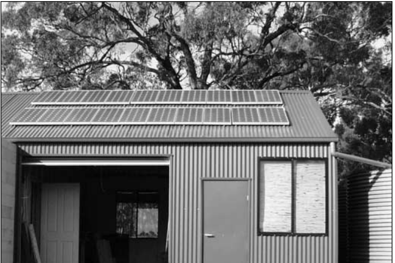
North facing solar modules on the roof collect energy.
