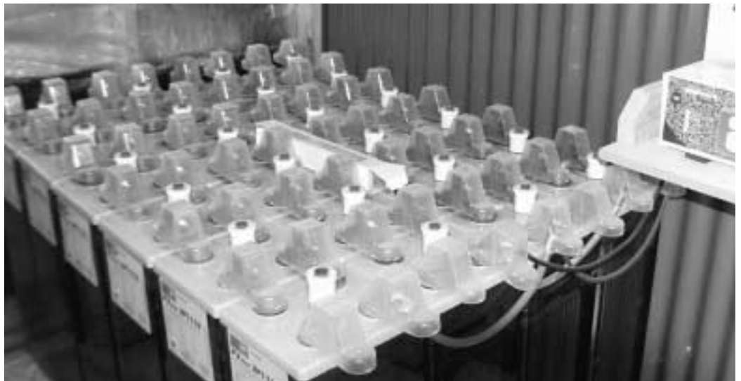
Renewable energy stored in high-cycle batteries.
